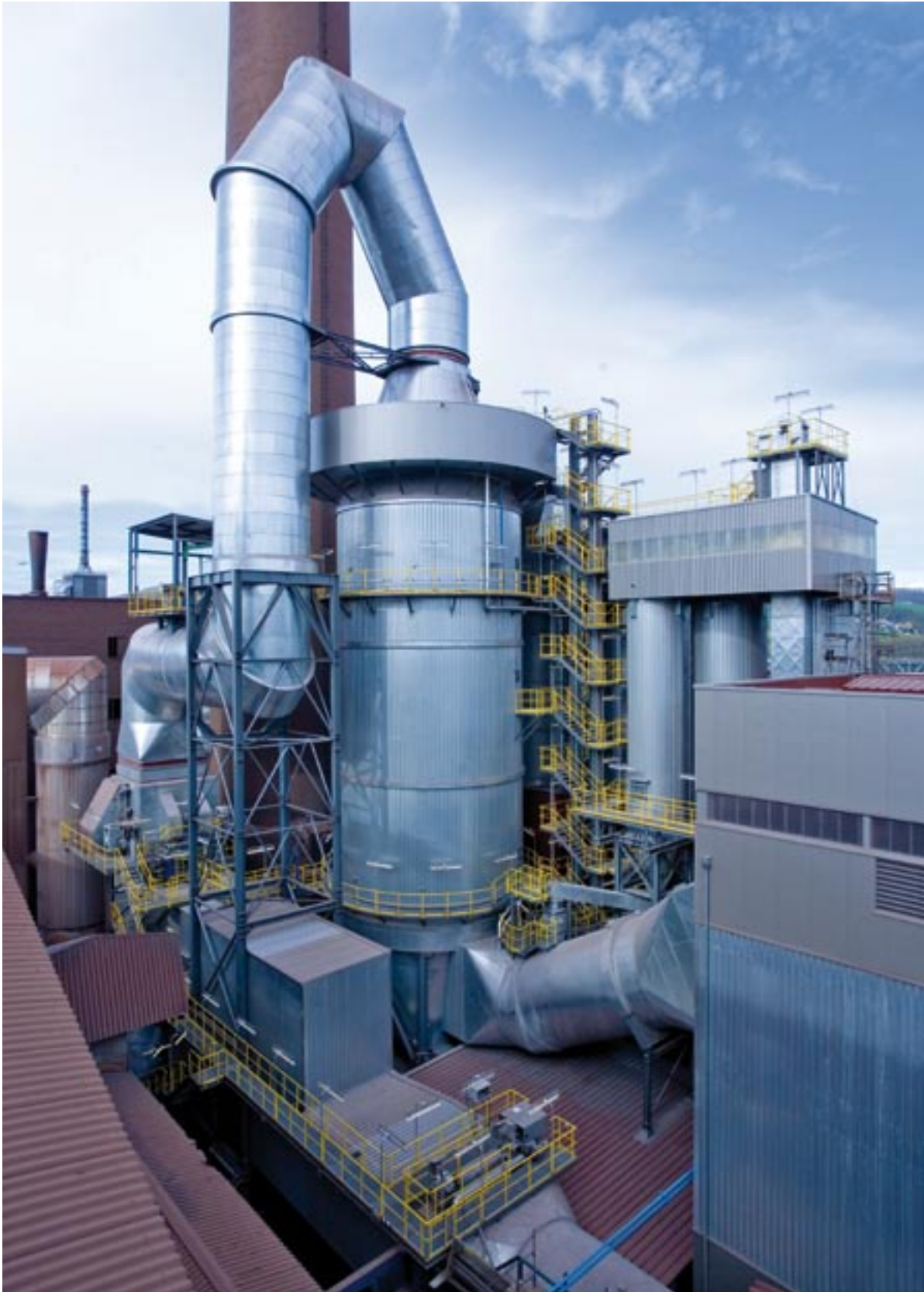
SIMETAL GS MEROS conditioning reactor and storage silos
